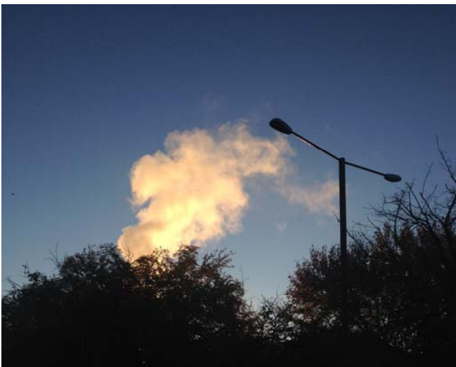
The new Satellite Chiller Plant on a winter morning - saving energy across campus
