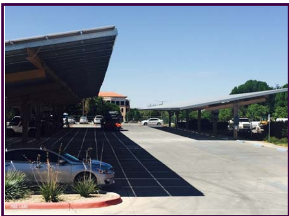
Solar covered parking in Lot 100
