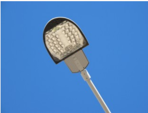
LED lighting installed on Geothermal Drive in 2010 reduces energy consumption and cuts energy costs
