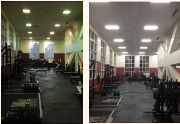
Before and after images of the lighting retrofit in the Activity Center weight room, which reduces energy costs, improves indoor lighting, and provides a monetary rebate from El Paso Electric
